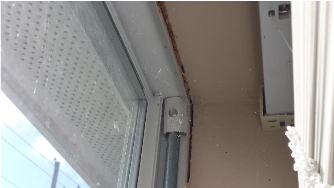
Note that there are separations between the window frames and the gypsum wallboard inside the window casings. Such separations are typically an indication of moisture inside the wall cavity.
