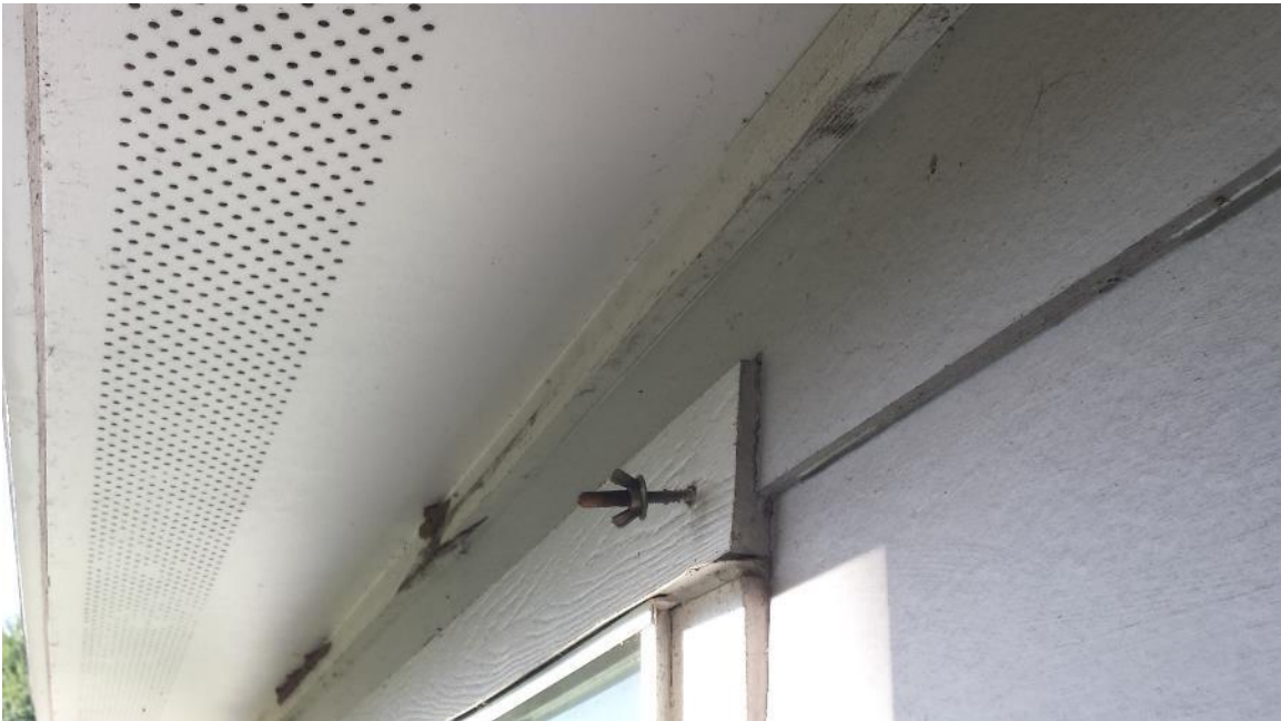
This is another view of the apparent termite damage on the outside of the front wall.
