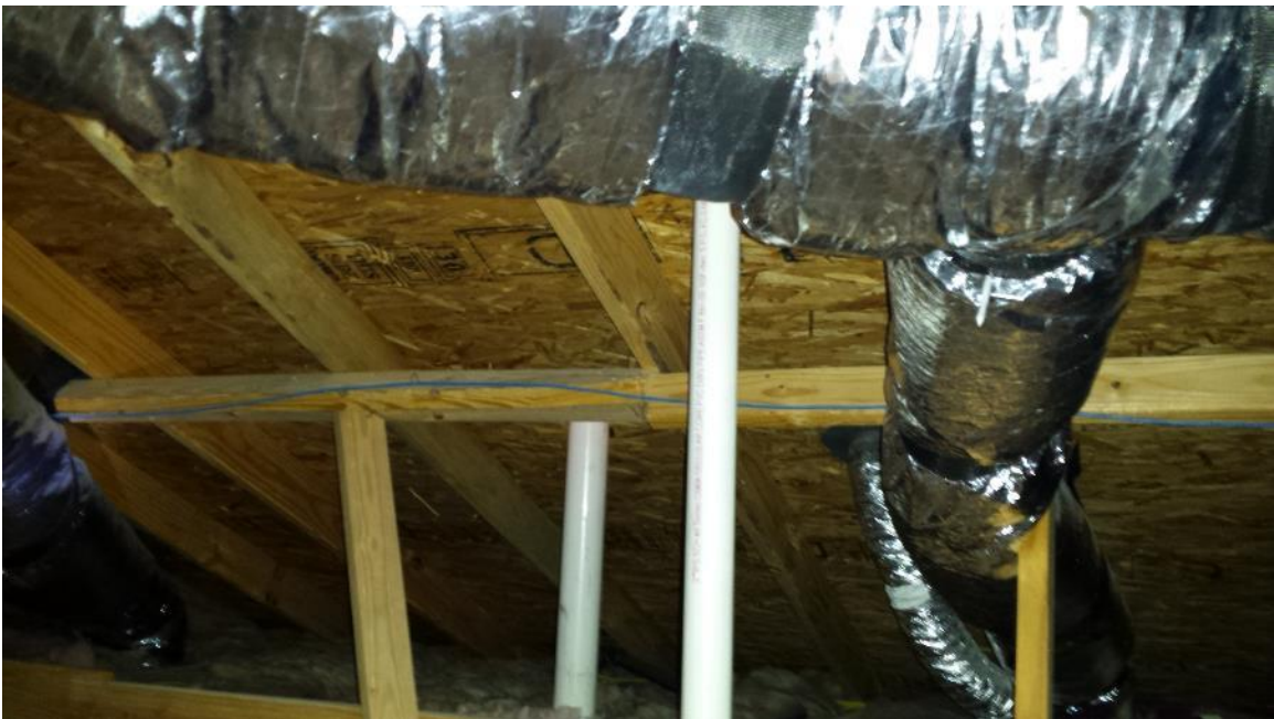
Here the purlins are not braced where they are spliced and are separating at this splice.
