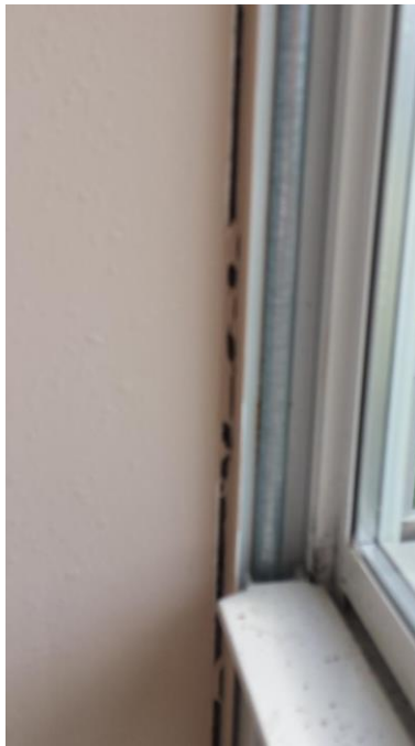
This is a view of additional separations between the window frames and the casings.
