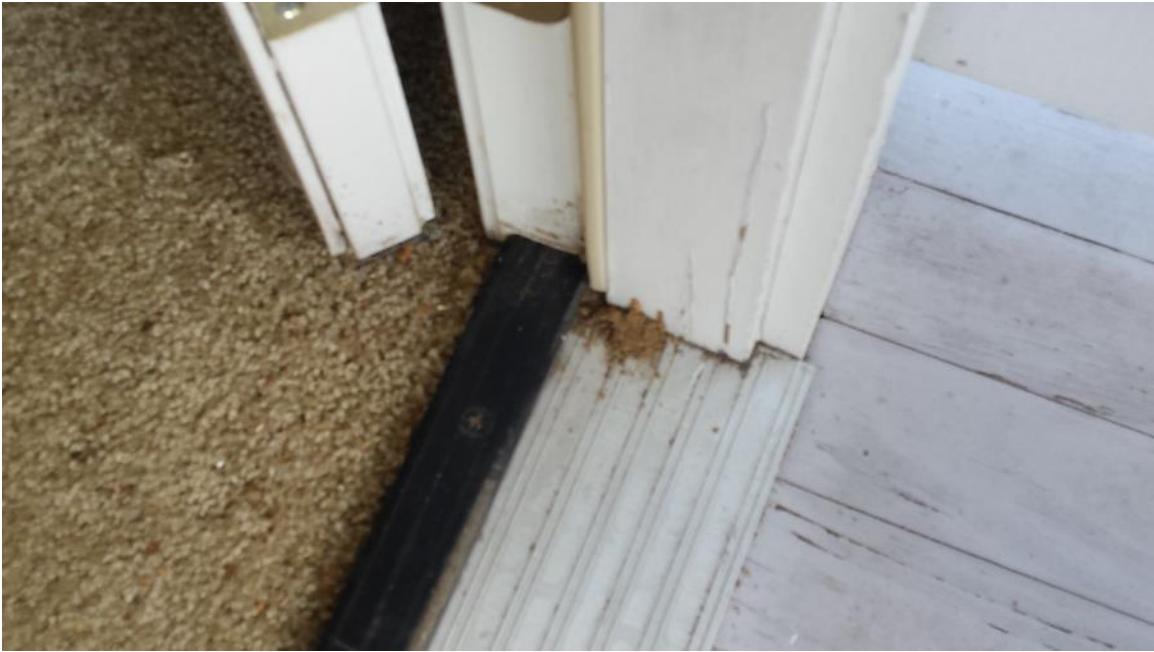
This is additional apparent termite damage at the front door threshold.
