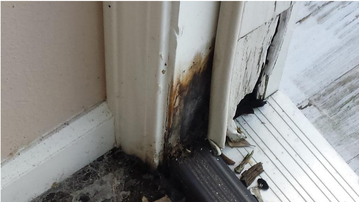
Note the water damage that is the result of leakage of the door and frame.
