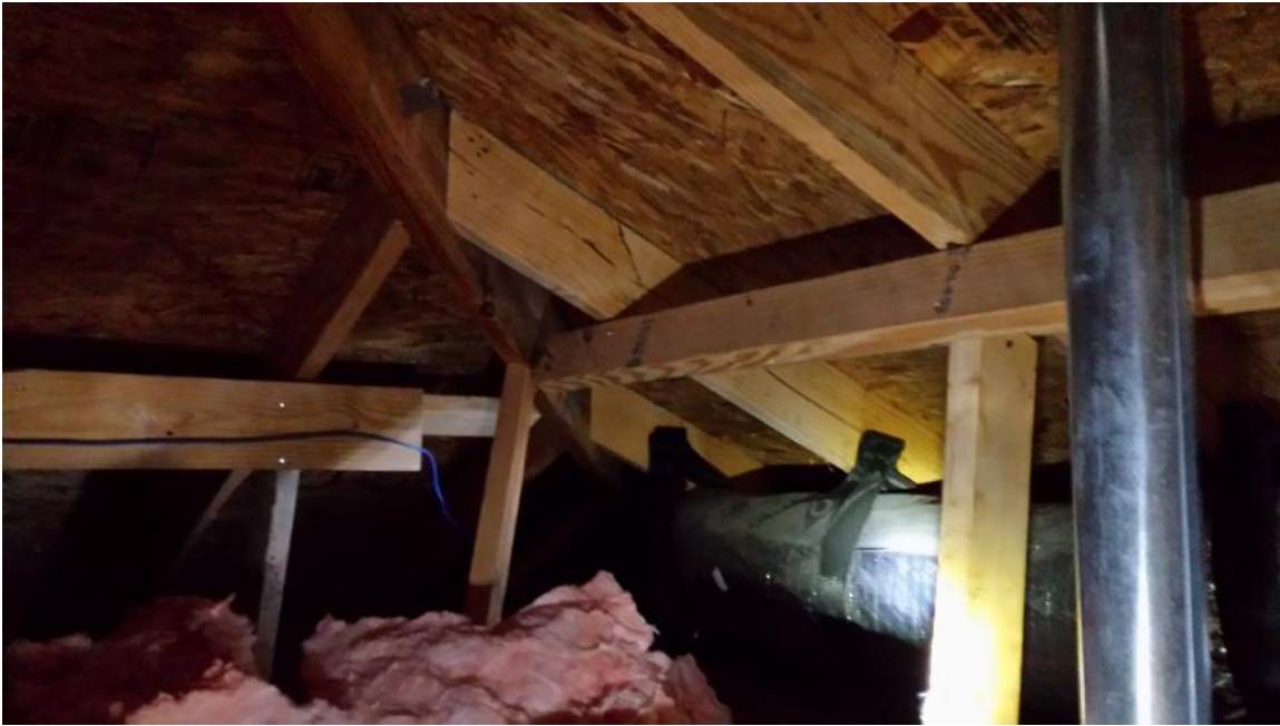
This end of the 2x4 brace is not supported and is deflecting visibly.
