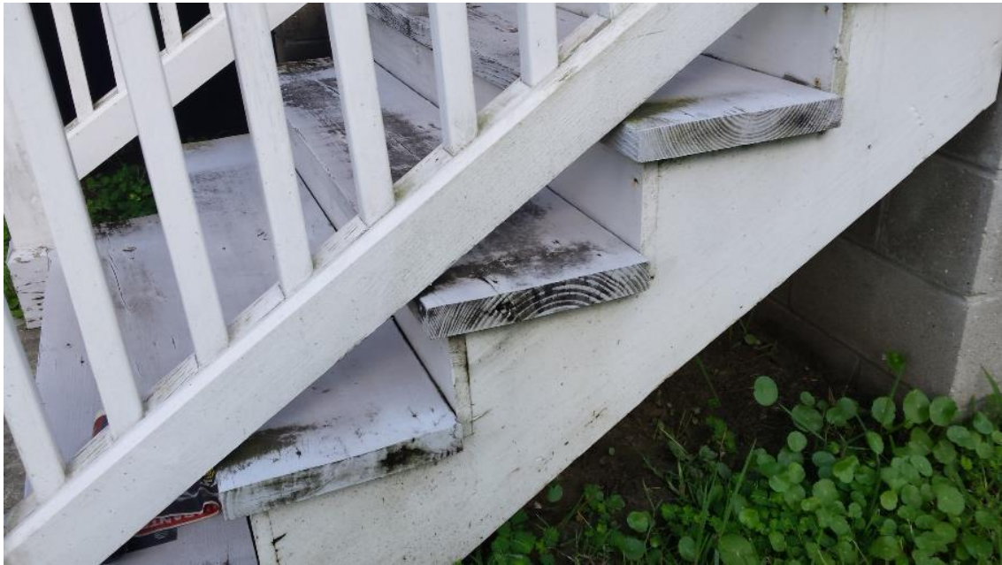
This is a view of discoloration and moisture effects noted at the front stair treads. In our opinion, this discoloration is premature and indicates that these treads were not sealed properly.
