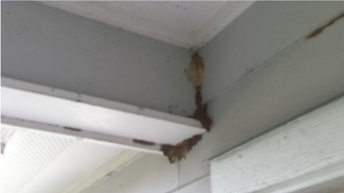
The evidence of apparent termite damage extends to the outside of the front wall of the house.
