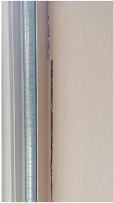
This is another view of the separations between the window frames and the casings.
