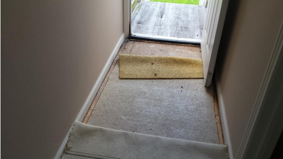
This is a view of the rear of the hallway at the rear door frame.
